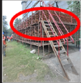
Handrail made from rejected boiler tubes
